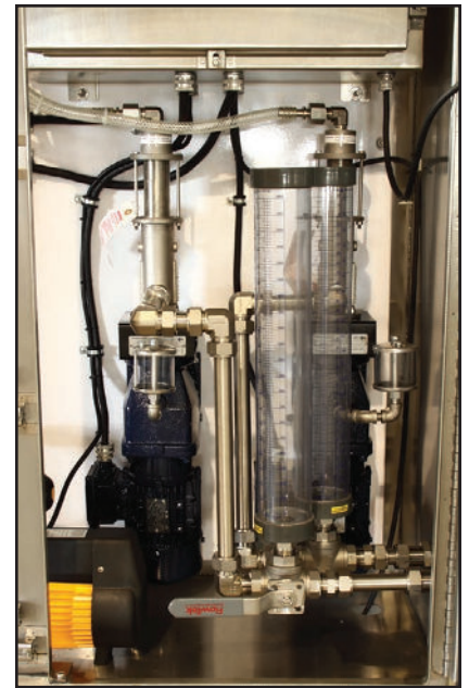
Figure 15 – Select Flocc™ Dual Polymer PC Feed Pumps
