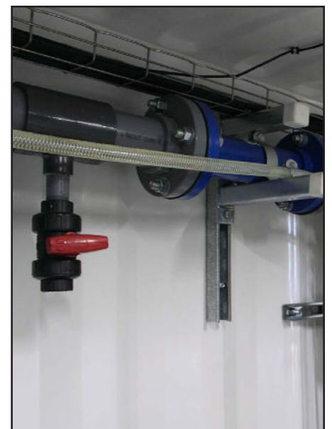
Figure 11 – Elgin's DFD Systems Incorporate InLine Static Mixers and Sampling Port.
