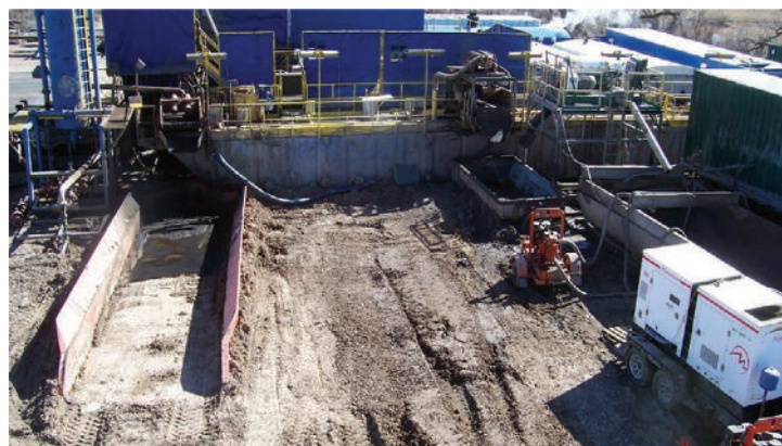
Figure 5 – Elgin's DFD System Using a Dry Reserve Pit.
