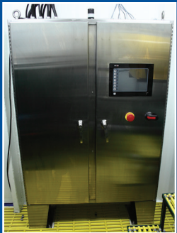
Cabinet Enclosure with Integrated Touch Screen Human Machine Interface (HMI)
