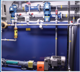
Dedicated Polymer Tanks with Top Mounted Agitators and Injection Pumps
